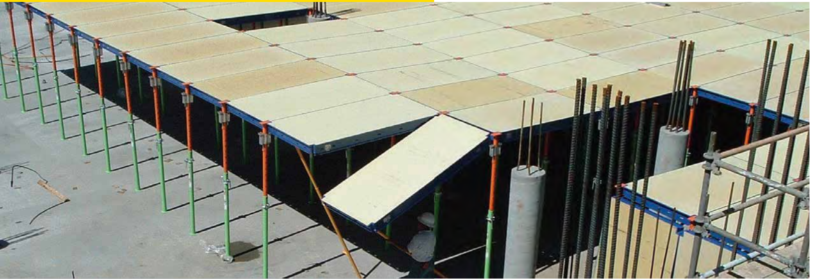
Panels, Props and ADT in use at a construction site in Washington.
