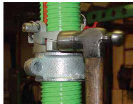
Step 8 Convert the lowest level of Props from backshoring to reshoring by striking the Quick Release above the Prop Collar. Release the load in the section as required by site Engineers. Allow the floor to "Take Up" self weight then snug up the Props.
